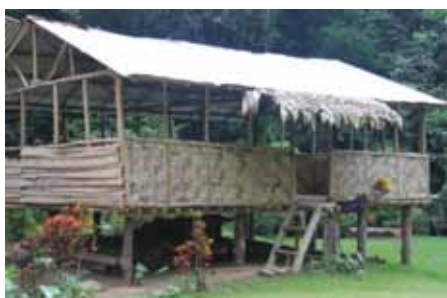
✓* Good ventilation, although lack of large eaves may allow rain inside.
