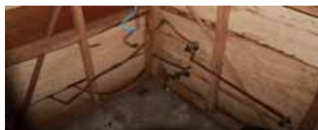
✘ Unfinished wiring/plumbing in bathroom. Unsafe and makes area unusable, even for a "bucket bath".
