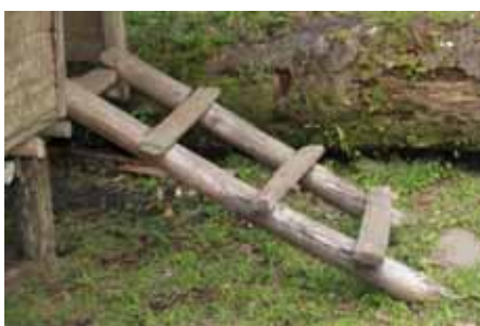
✘ Step slope too low.
