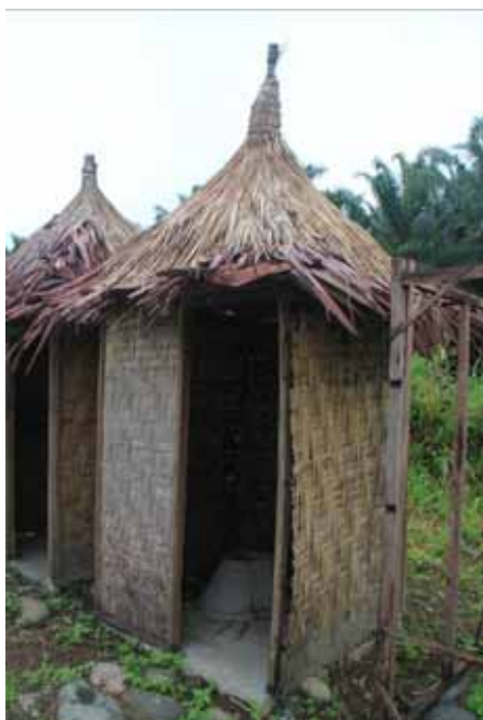
✓✗ .No door, concrete pedestal difficult to squat at or sit on.
