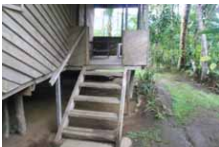
✓ Very good steps, well spaced, good bottom landing stone, just needs an outer handrail!
