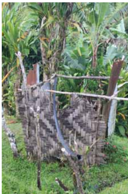
* Rotting wall matting detracts from an otherwise spectacular view.
