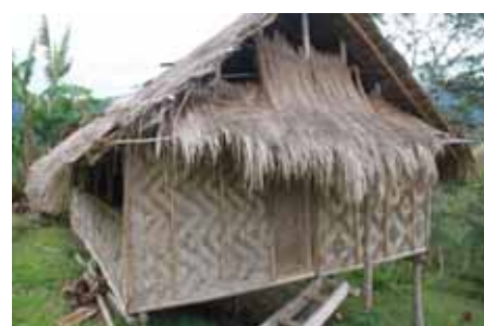
✘ Steps do not have a landing and do not match the door.
