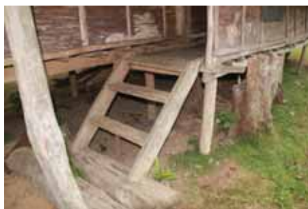
✓* Sturdy, bottom landing, good slope, good height. Could use a hand rail, but not essential for this height.
