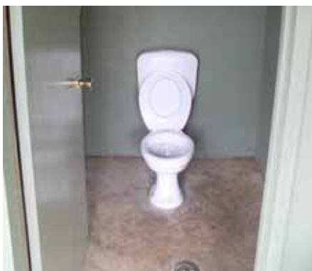
✓ Normal flush toilet at Oro Haven
