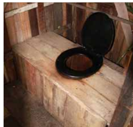
✓ Timber box pedestal.
